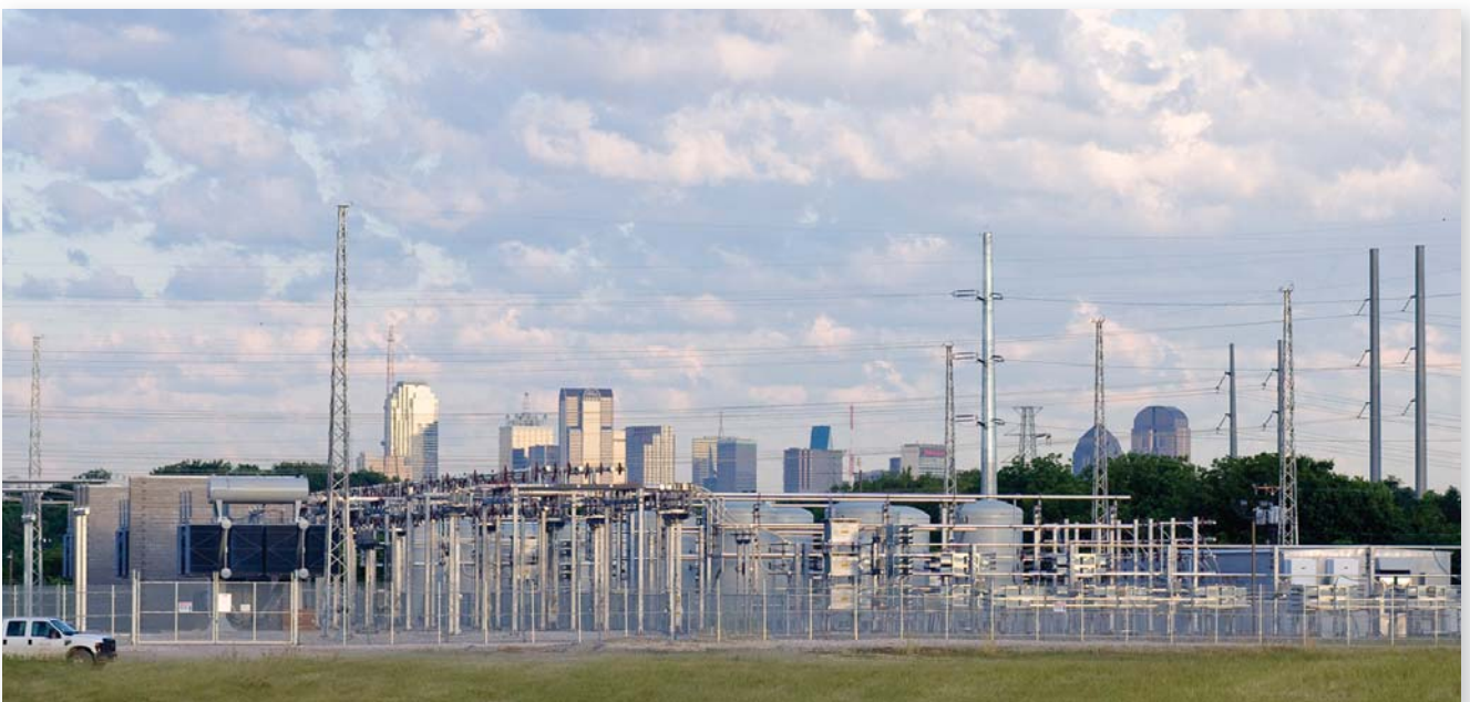
Oncor has installed the world's largest concentration of Smart Grid voltage compensation equipment, static VAR compensators, in Dallas.
