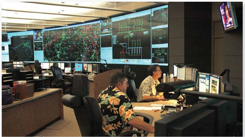
Oncor's Gary Moody and Chris Parker work at Oncor's Transmission Grid Management center, a facility that never sleeps, constantly monitoring flow of electricity through more than 15,000 miles of transmission lines.
