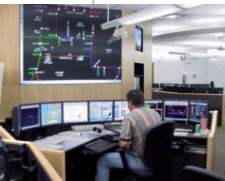
Fig.3 - PROGRESS ENERGY - SALA CONTROLLO
